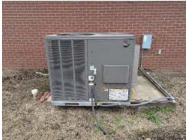
Figure 3: 5-Ton Rheem Unit
